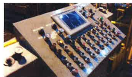
TYPICAL CONTROL CONSOLE
